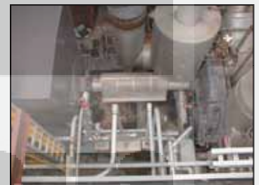
Compressor at wastewater plant
