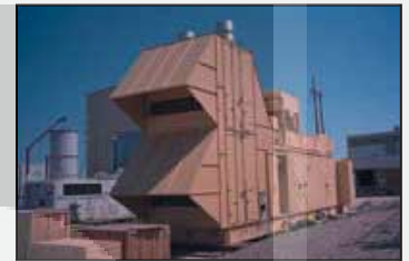
Gas turbines at co-Generation facility
